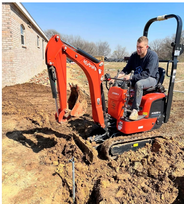
Hardin’s Family Plumbing is now serving a growing client base, with initial support from the Citizen Potawatomi Community Development Corporation. (Photo provided)
