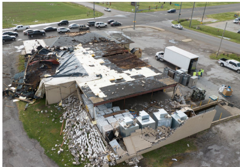
The former Hardesty Grocery Store suffered major damage following the April tornado.
