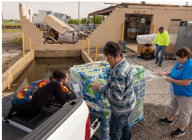
Employees cleared out the heavily damaged former Hardesty Grocery Store following the tornado.
