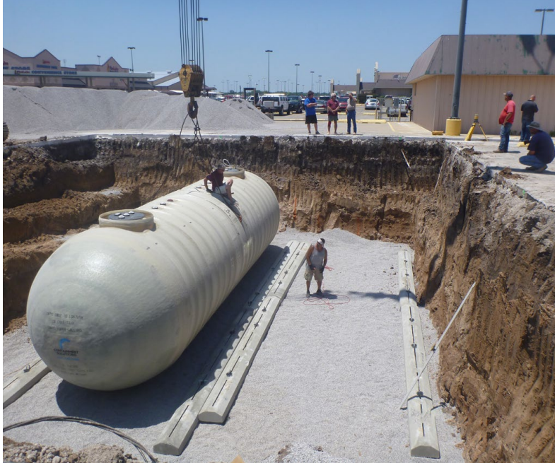
Crews install underground storage tanks at FireLake Corner Store in 2013. (Photo provided)
