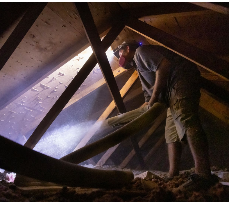
A volunteer blows insulation into an attic during weatherization improvements for units in Father Joe Murphy Elder Housing.
